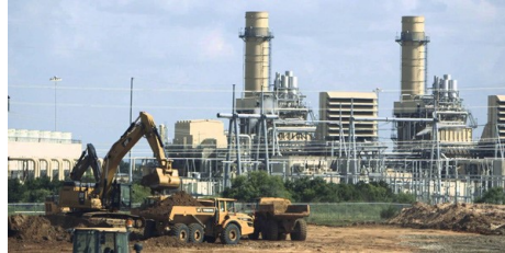
The 738-MW Wolf Hollow facility in Granbury, Texas, is one of the four power plants in the state Exelon will sell as part of the bankruptcy of its ExGen Texas Power subsidiary. | GE Power
